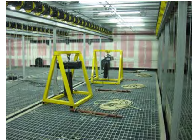
Wide angled photograph of a grate style grid floor with typical pulley arrangement.
