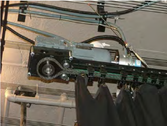
Motor driven track and drape
