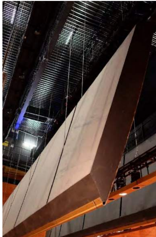
Example of a permanent adjustable acoustic canopy suspended from steel wire ropes
