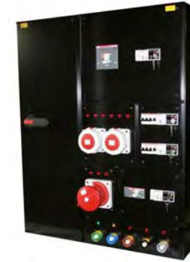
Typical custom temporary power panel
