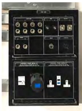
Typical audiovisual facilities panel
